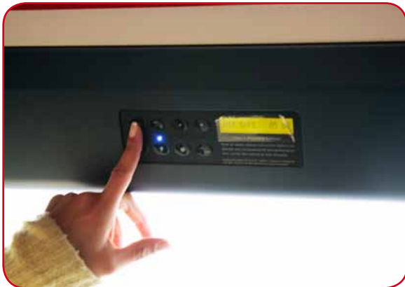
3. Check that all functions of the BSC / UAC are regular
